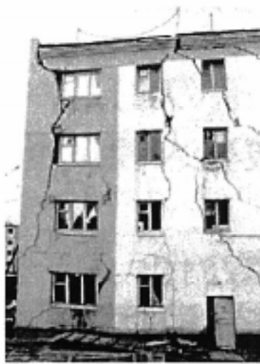
Building damaged due to permafrost thawing in Chersky (low Kolma River), Russia.
