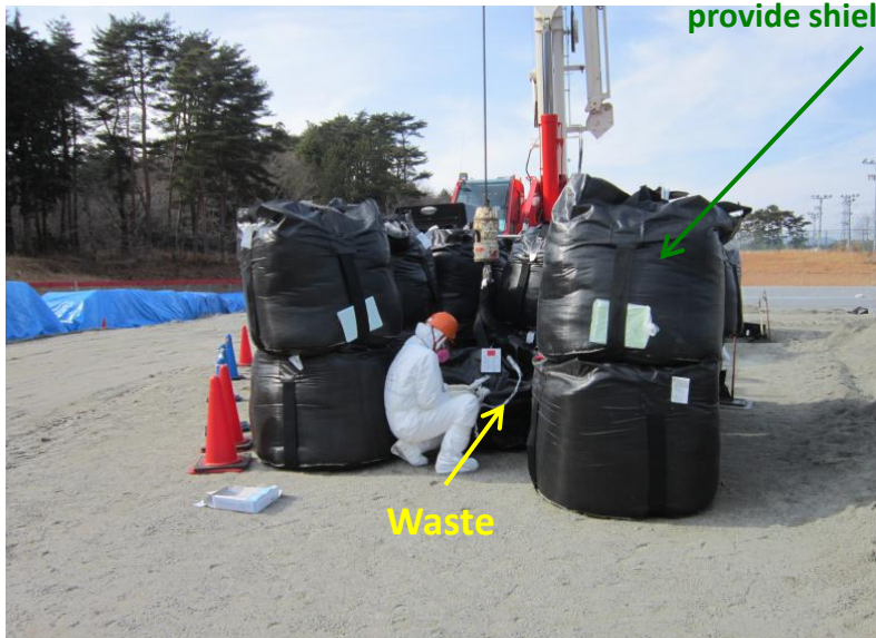
Measurement of surface dose rates of decontamination waste in the shielding zone
